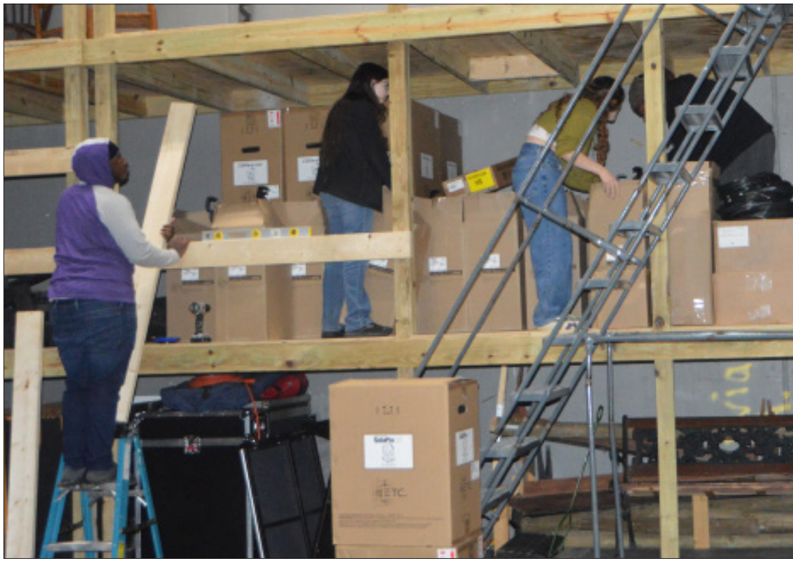
Theater tech students build a shelf to store construction resources on. Construction started in October and is expected to last several more months. • PHOTO BY NICO JORDAN
